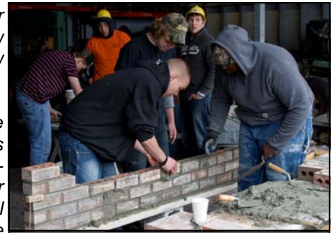
A group of students build a brick wall during one of the hands-on activities.
